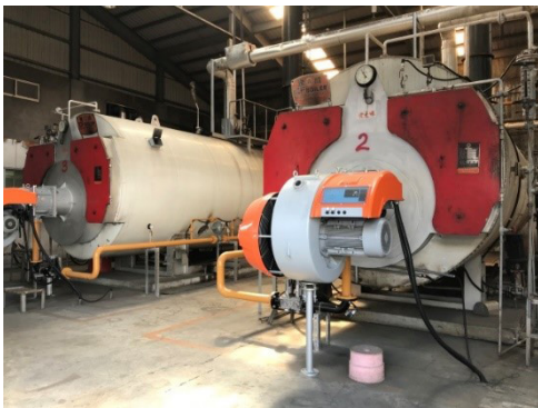
▲ Modified combustion engines of boilers
